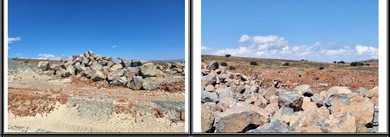
CONCRETE BATCHING AREA
