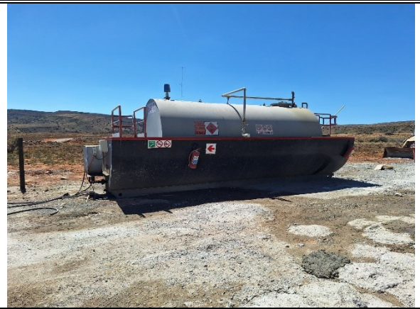
WATER TANK FOR CONCRETE MIXING
